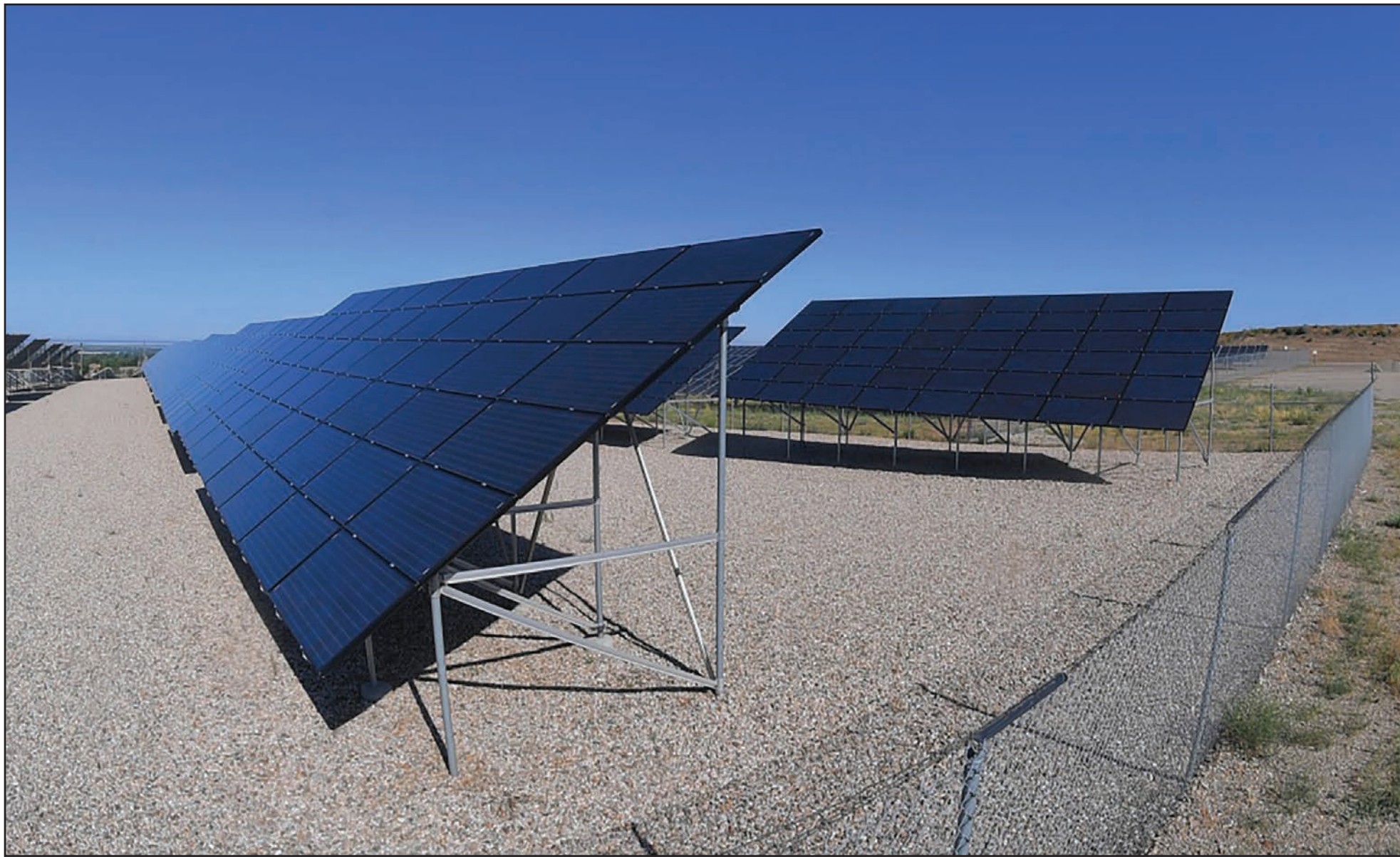
Construction of a new 3.55-megawatt solar array was completed last summer at Hill Air Force Base as part of a $42 million upgrade project. The array feeds directly into the electric grid, adding to the base's existing renewable energy production capability and
