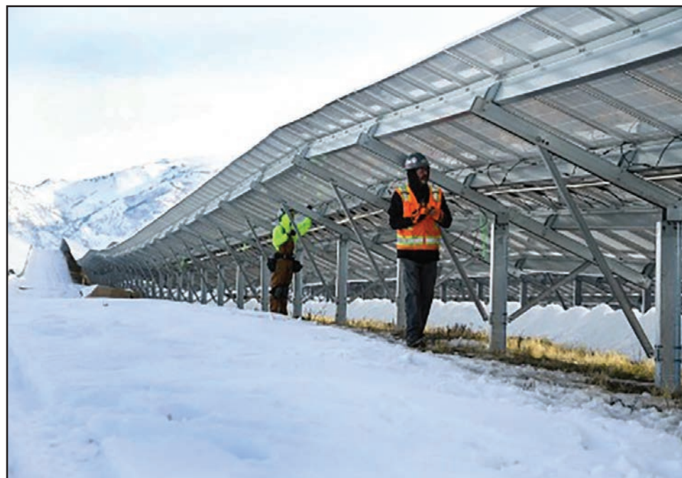
Technicians complete work on a 3.55-megawatt addition to the solar panel array at Hill Air Force Base. (U.S. Air Force photo by Todd Cromar)
